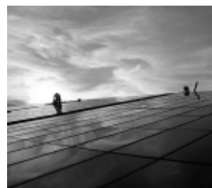
Solar panels on the Cambria Office Building of the Pennsylvania Department of Environmental Protection. Picture courtesy of NREL/DOE.
